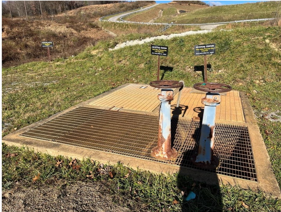
Photograph 3. West Valley Leak Detection and Leachate Collection Box.
