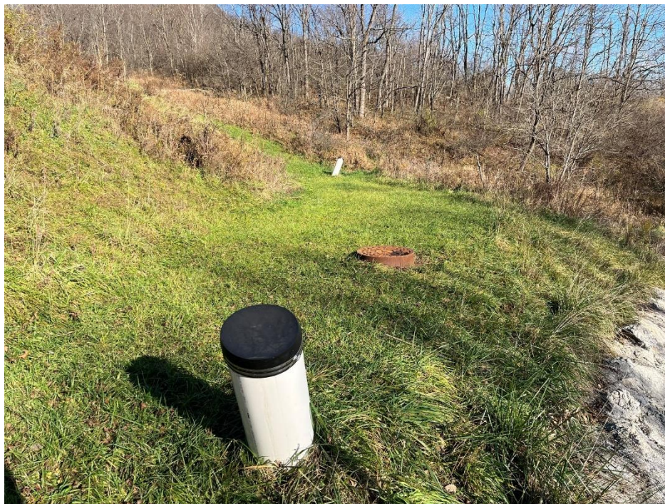
Photograph 7. View of East Valley Toe Bench and Leachate Seep Collection Pipes and Cleanouts added in 2019, view north.
