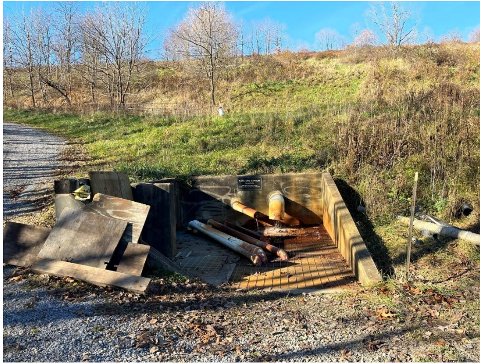
Photograph 5. East Valley Leachate Collection Box, view west.
