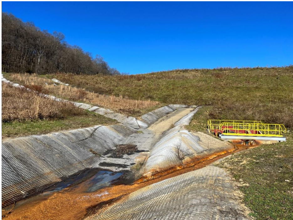
Photograph 4. Stage IIIA toe collection channels and leachate and leak detection flows from stilling basin (right); view north.
