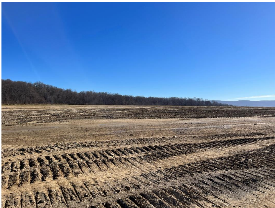
Photograph 15. The northern-most top area of Stage II, intermediate cover placement; view east.
