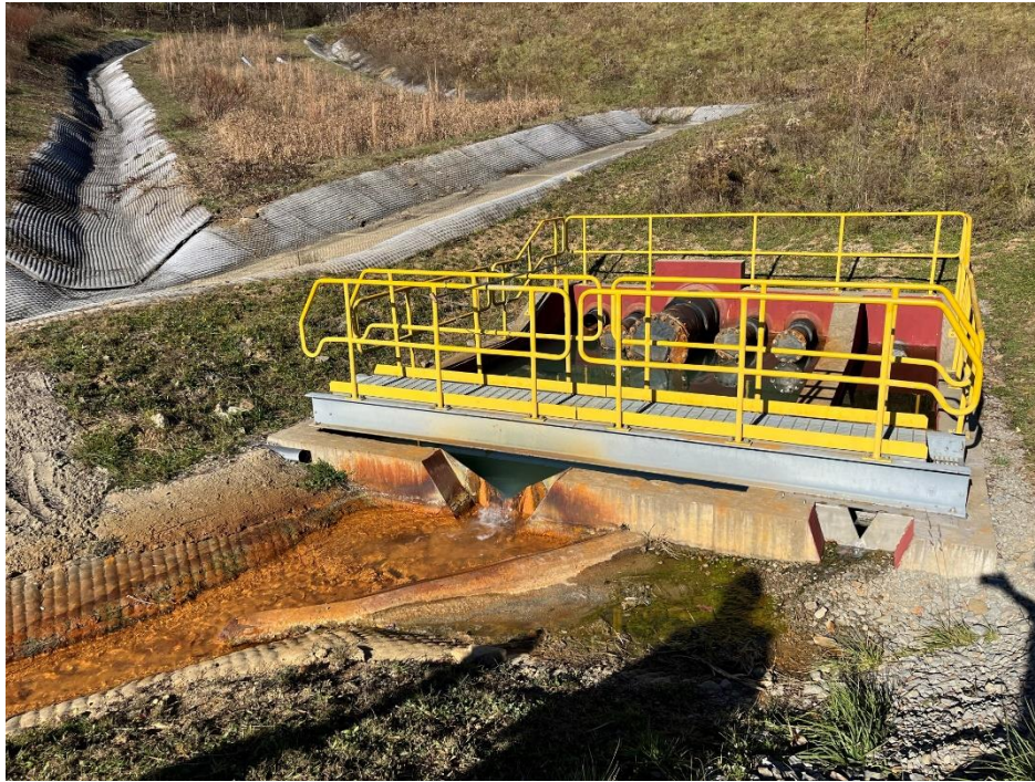
Photograph 3. Stage IIIA Stilling Basin, Leachate collection piping and v-notch weir (left), Leak detection pipe and v-notch weir (right).
