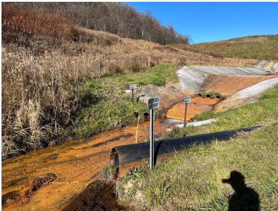
Photograph 5. Stage IIIA toe collection channel and flows from subgrade drainpipes (with signs) from Stages II/III; view westward.
