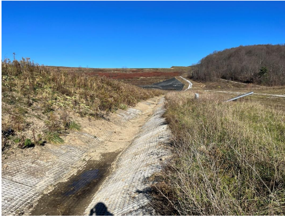
Photograph 7. Stage IIIA Collection Channel along first bench on east side of Stage IIIA; view northeast.
