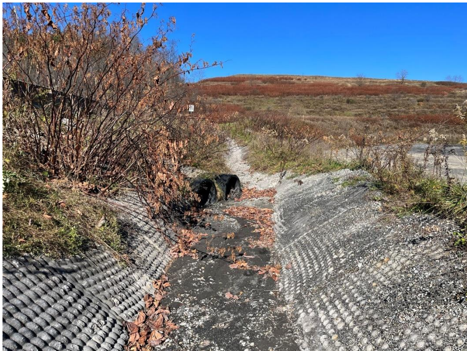
Photograph 26. Haul road collection channel and culvert to be cleaned of sediment build up; view north.
