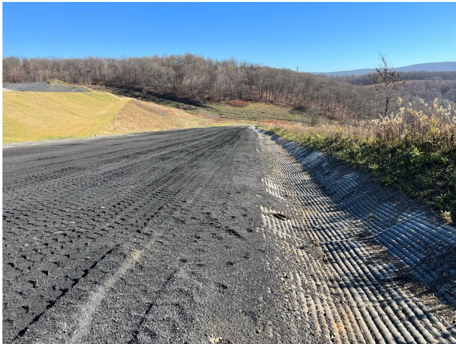
Photograph 18. Stage II active disposal area (left), haul road (center), and haul road drainage channel (right); view east.
