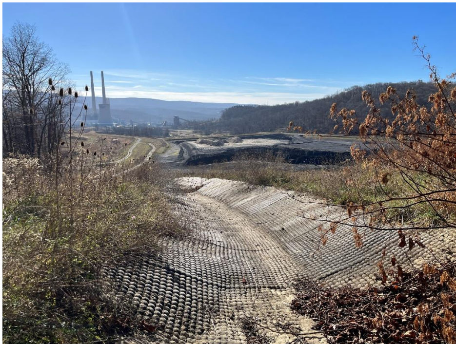
Photograph 10. East Side Collection Channel (foreground) and active Stage IIIA (background); view south.
