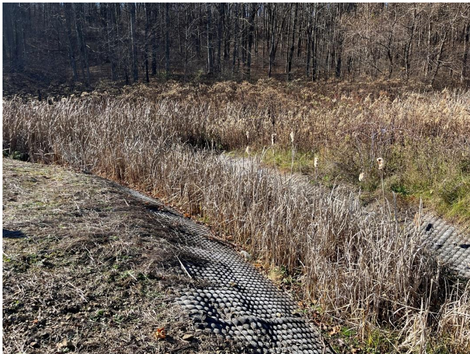
Photograph 24. West Diversion Channel, adjacent to Stage IIIA, along the Stage II haul road, to be cleaned of sediment build up; view south.
