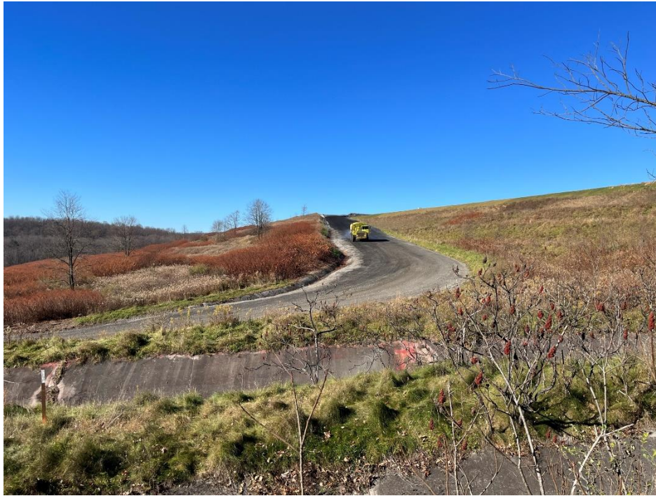
Photograph 9. Water truck, providing dust control on haul road to Stage II; view west.
