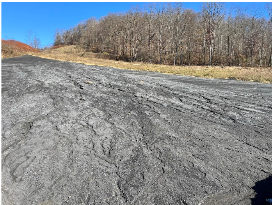
Photograph 8. Erosion rills to be monitored and repaired as necessary in the northeast corner of Stage IIIA.
